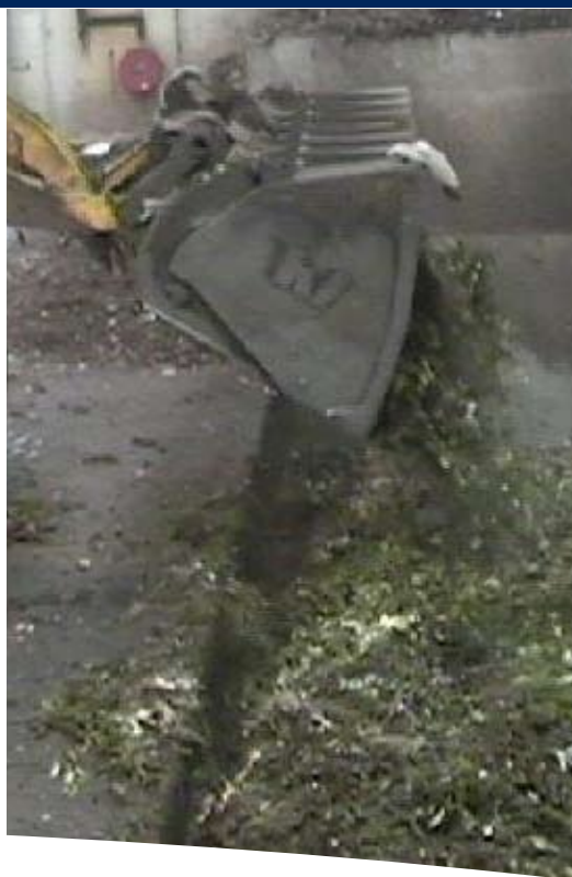
Spiro Conveyor Floor build into a concrete pit Spiro-Schubböden in einer Betonrinne
